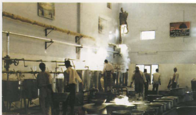
A view inside one of the kitchens of the world's largest solar cooking facility at Brahma Kumaris Shantivan campus, Abu Road
